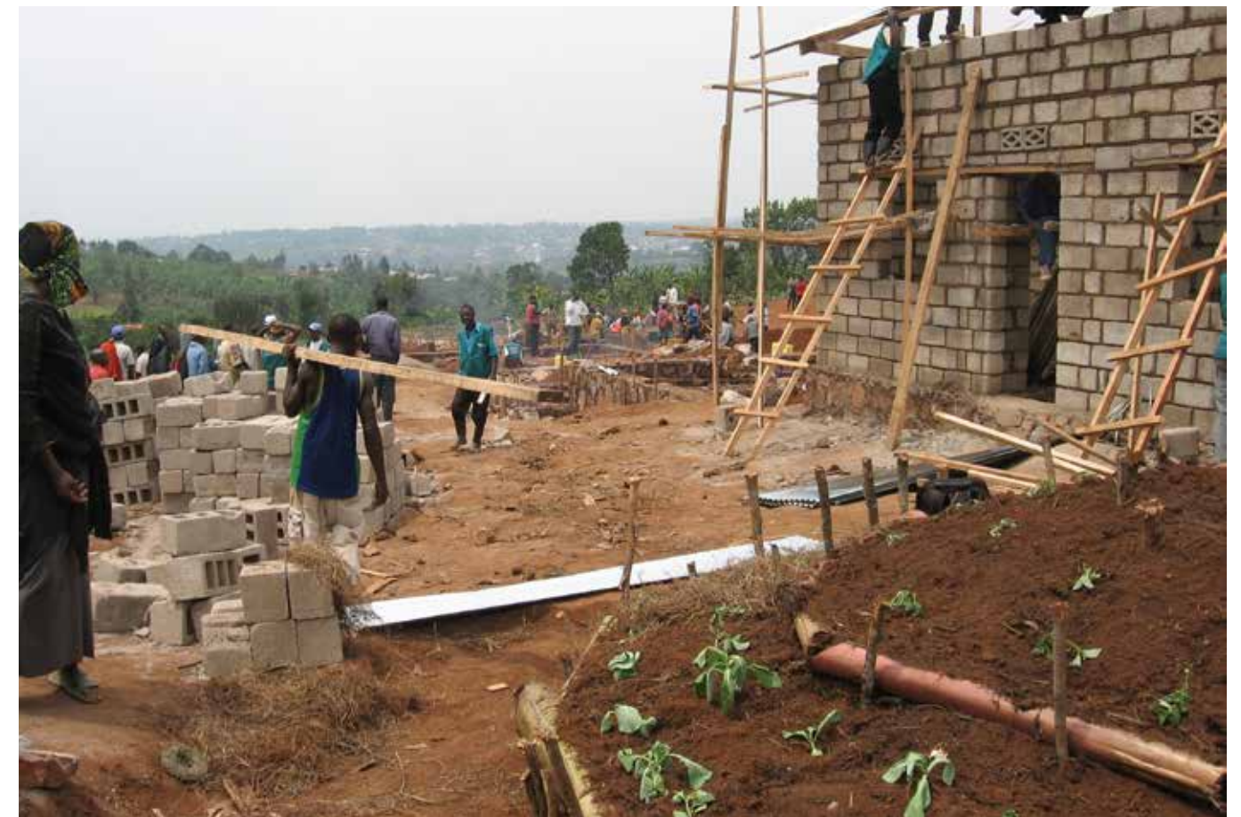
In 2011, the Batwa community at Bwiza—including members of Kwizera—moved to newly built homes provided by the government at Cyaruzinge (shown here under construction). At the official launch of the new housing, members of Kwizera had the honor of performing for Rwanda's First Lady. Photo: Phil Vernon, 2011
